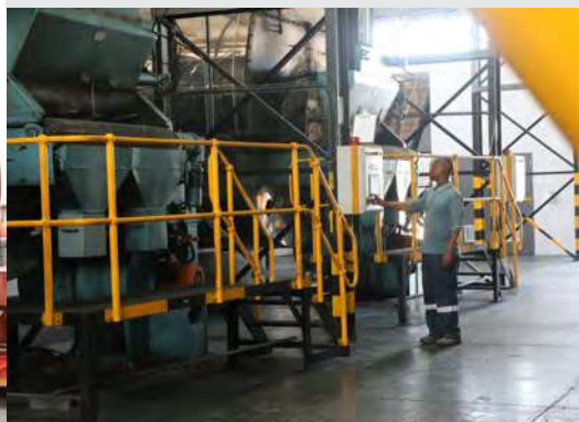
Boiler House Management
